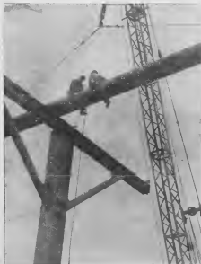
The first of the overhead pipeliners to feed the new East Finger Pier goes up as men of Chicago Bridge talk over the job from a perch high above the ground. The huge sections of pipe were raised into position by the crane, background, and then secured to each of the big T-trusses. The lines run at a height of 40 feet for a distance of 154 feet before bending down, left, to feed into the pier.
